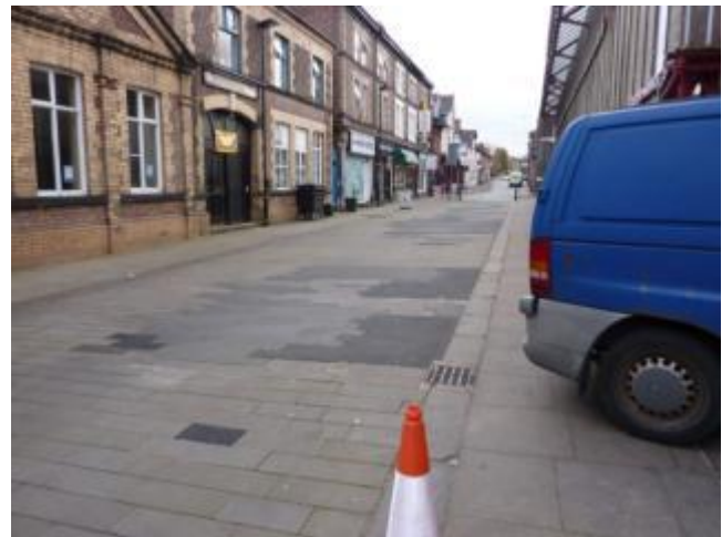
Photograph 98: Poor Street Surface to Greenwood Street
