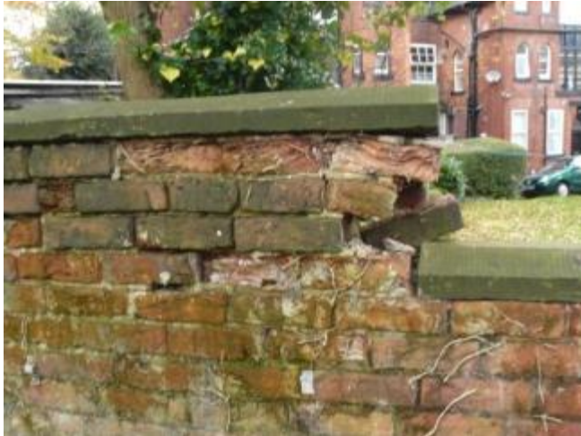
Photograph 93: Spalled brick boundary wall to Church
